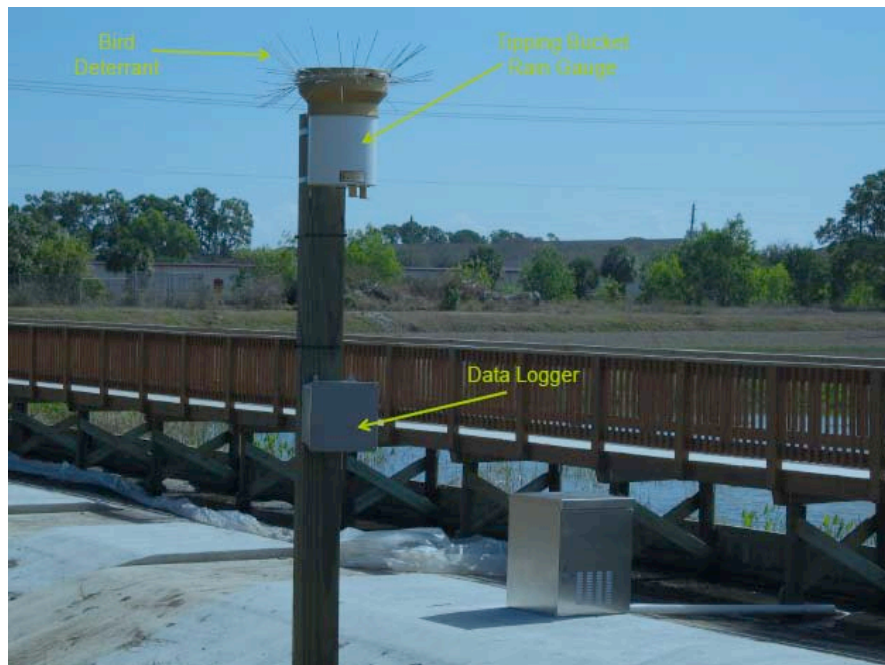
Figure 6, Outfall Autosampler on Weir
