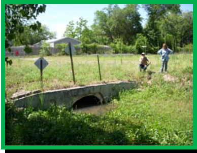
Existing outfall from County Pond into existing swale at Echo Circle Site
