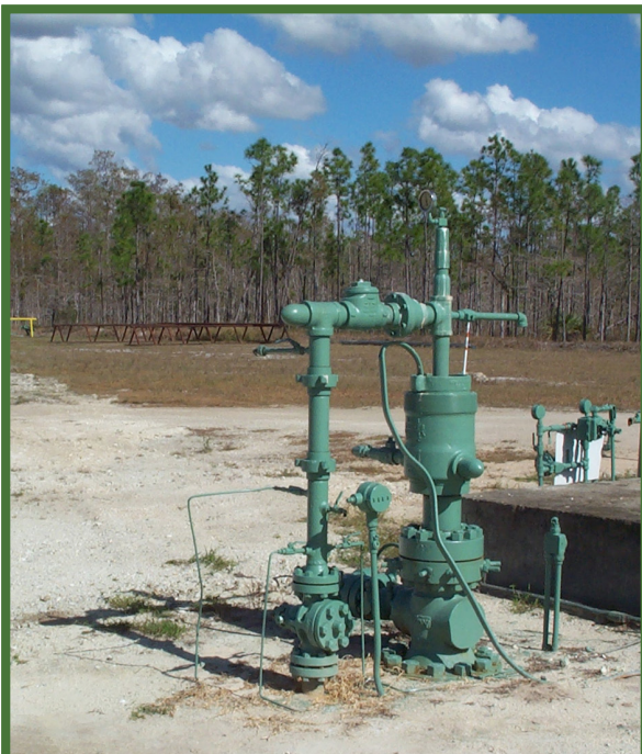
Typical southwest Florida oil production well with downhole electric pump, Raccoon Point
