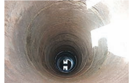
View into a hand-dug well cased with concrete rings; Ouelessebougou, Mali.
