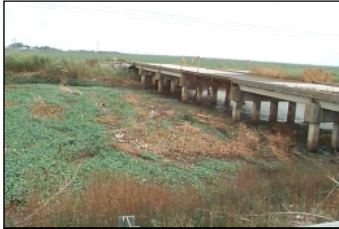
Trash and weeds trapped behind a bridge over the West Palm Beach canal.
