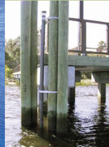
Water quality monitoring station attached to a piling
