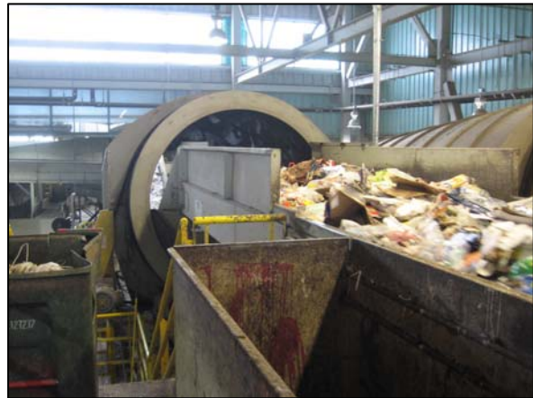
Figure 3.18: Trommel Screen at WPWMA
