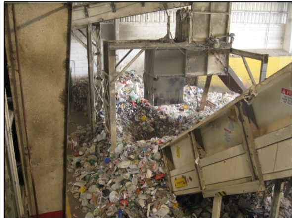
Figure 3.1: In-feed Conveyor at Orange County MRF
