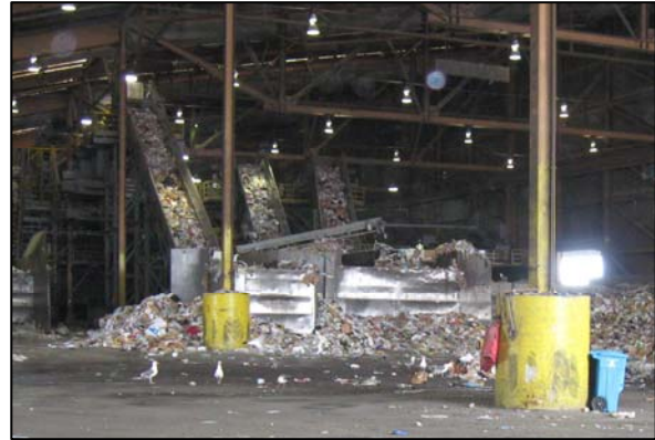
Figure 3.7: In-feed Conveyors at Pier 96
