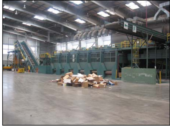
Figure 3.25: Puente Hills MRF Line
