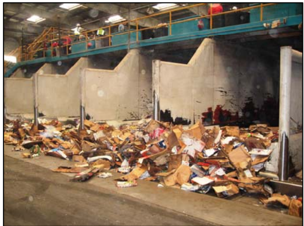
Figure 3.17: Storage Bunkers and In-floor Conveyor to Baler
