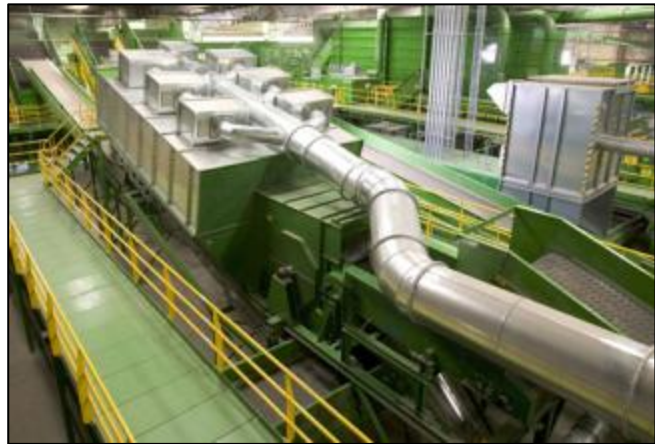
Figure 2.9: Air Drum Separator
