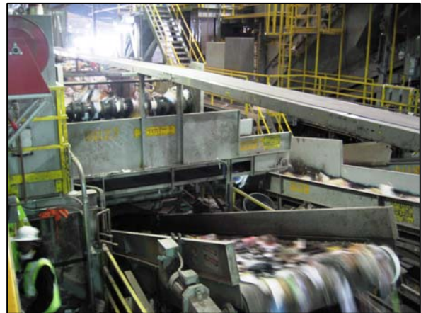
Figure 3.8: Disk Screen at Pier 96 with Top Conveyor Running Above
