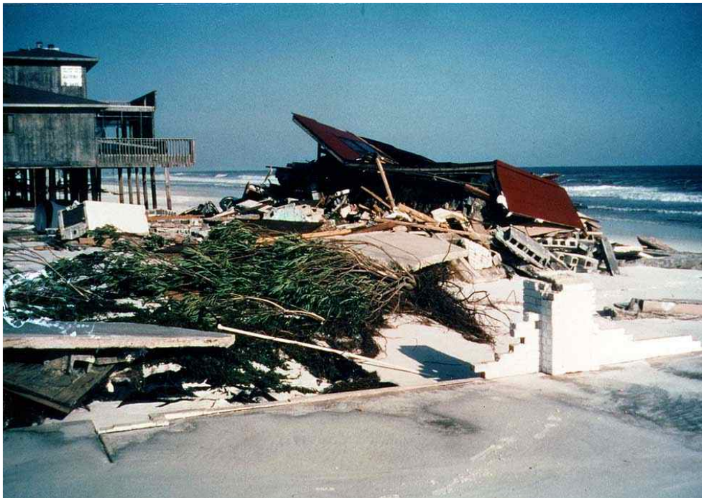
Figure 58. Escambia County - Pensacola Beach. This shows the contrast between a pile-supported structure which survived Opal and a poorly-designed one which did not.
