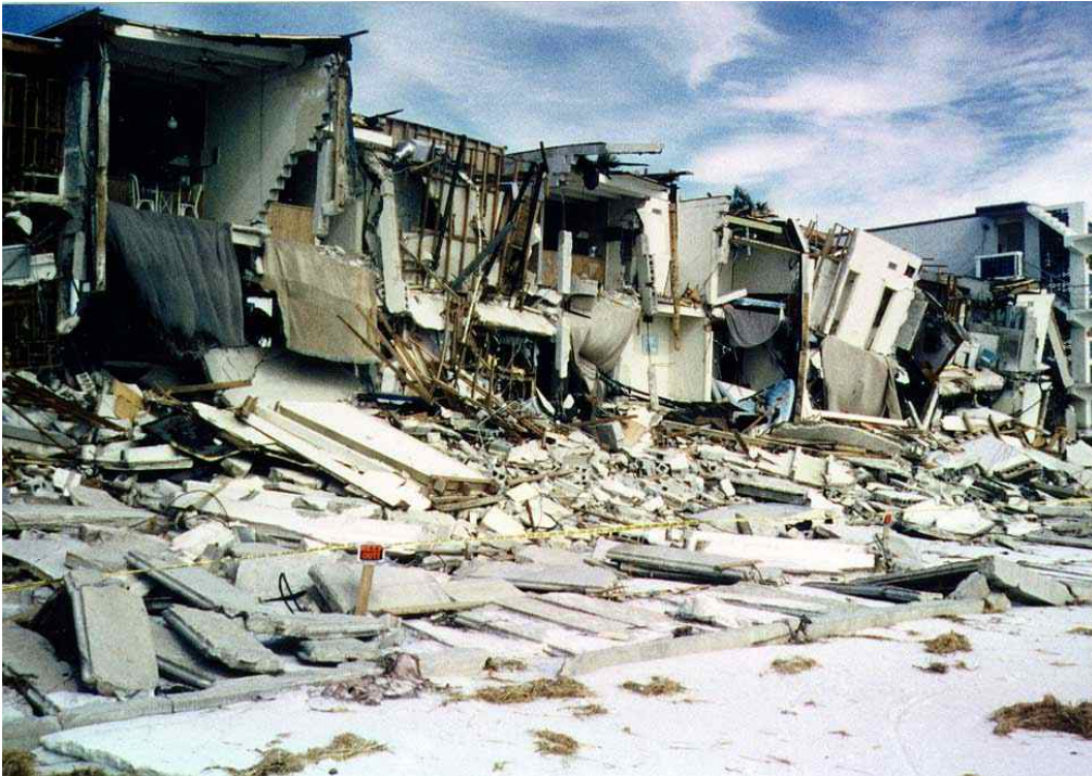
Figure 60. Bay County - Panama City Beach. This shows a seawall which was destroyed and did not protect the severely damaged multi-family dwelling from Opal.
