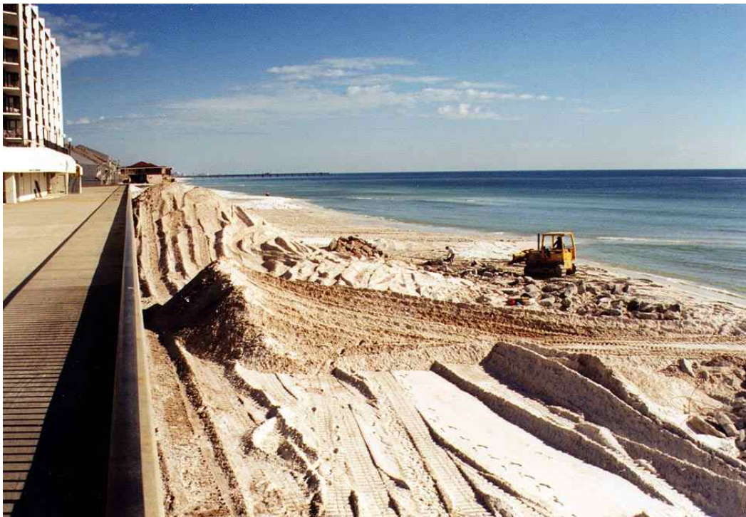
Figure 65. Typical Beach Scraping Along Panhandle After Hurricane Opal
