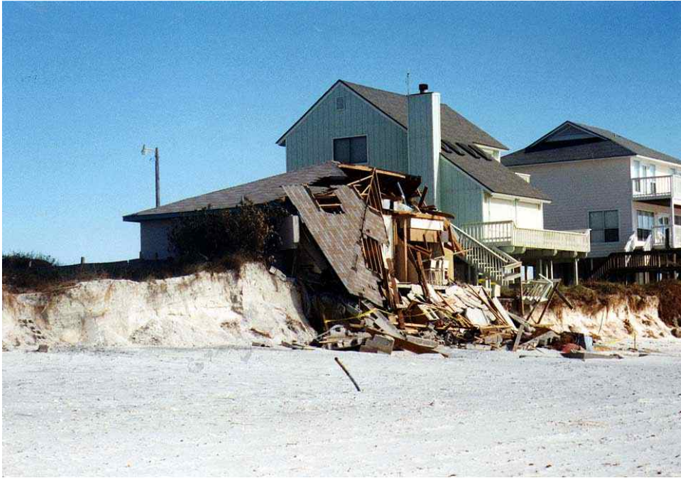
Figure 61. Gulf County - St. Joseph Peninsula. Poorly-sited and poorly-designed structure destroyed compared to permitted structures with better siting and design.
