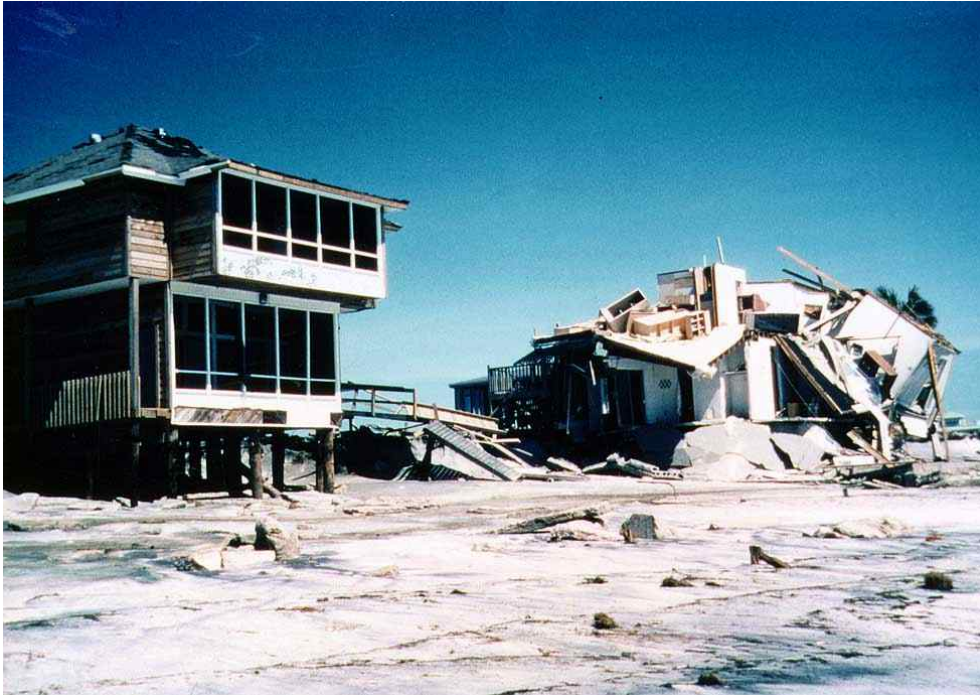
Figure 59. Walton County - Dune Allen. Contrast between a pile-supported structure which survived Opal and a poorly-designed one which did not.
