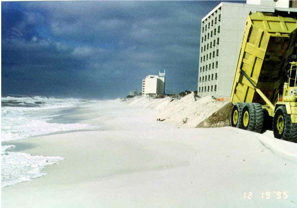
Figure 77. Redistribution of recovered overwash sand trucked back to eroded dune areas following Hurricane Opal in the Pensacola Beach area.
