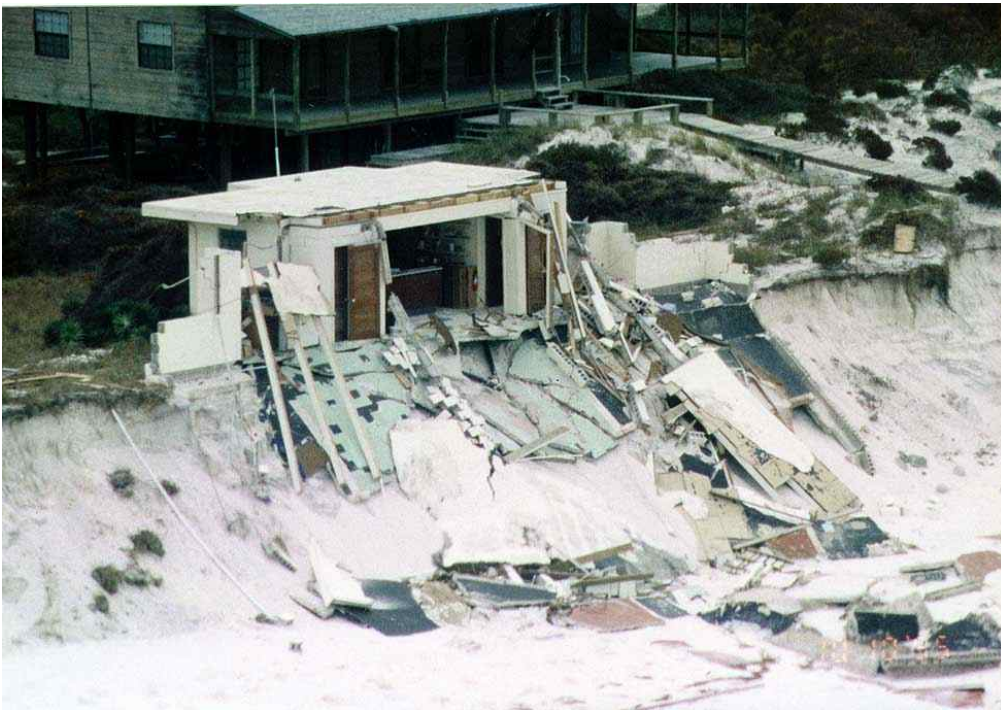
Figure 62. Franklin County - Dog Island. Major habitable structure with poor siting destroyed, over 150 miles from the point of landfall of Hurricane Opal.
