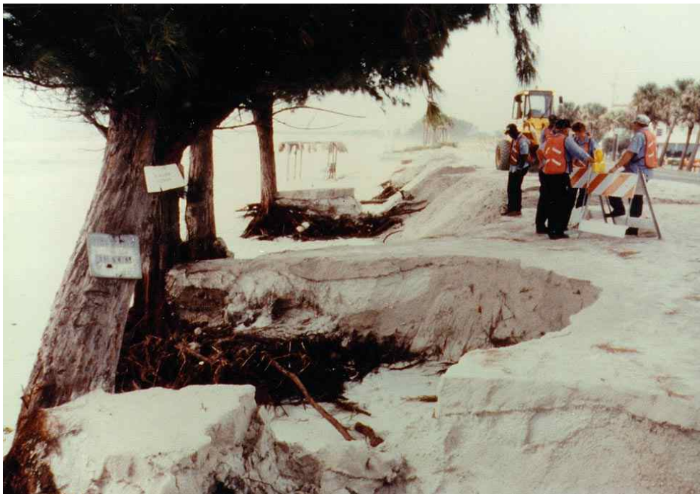
Figure 50. Erosion of beach restoration project on Longboat Key from Opal.
