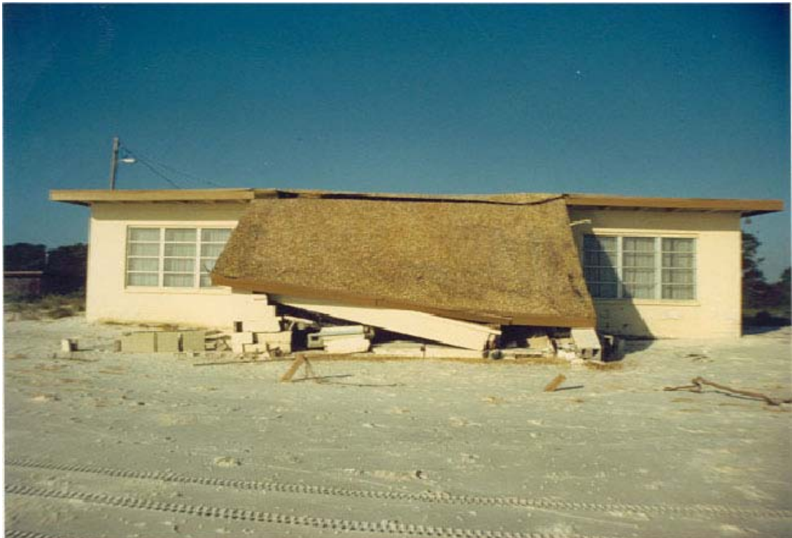
FIGURE 98. Wave damage to dwelling near Bald Point.
