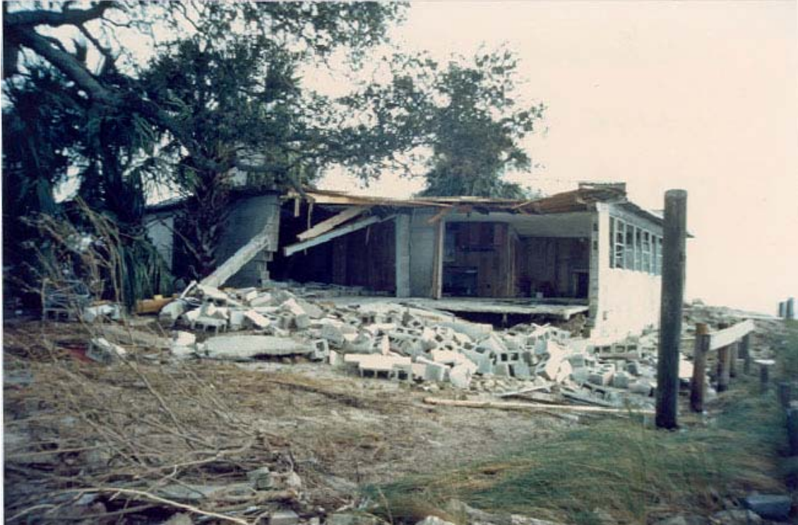
FIGURE 113. Dwelling destroyed at west point of Live Oak Island.
