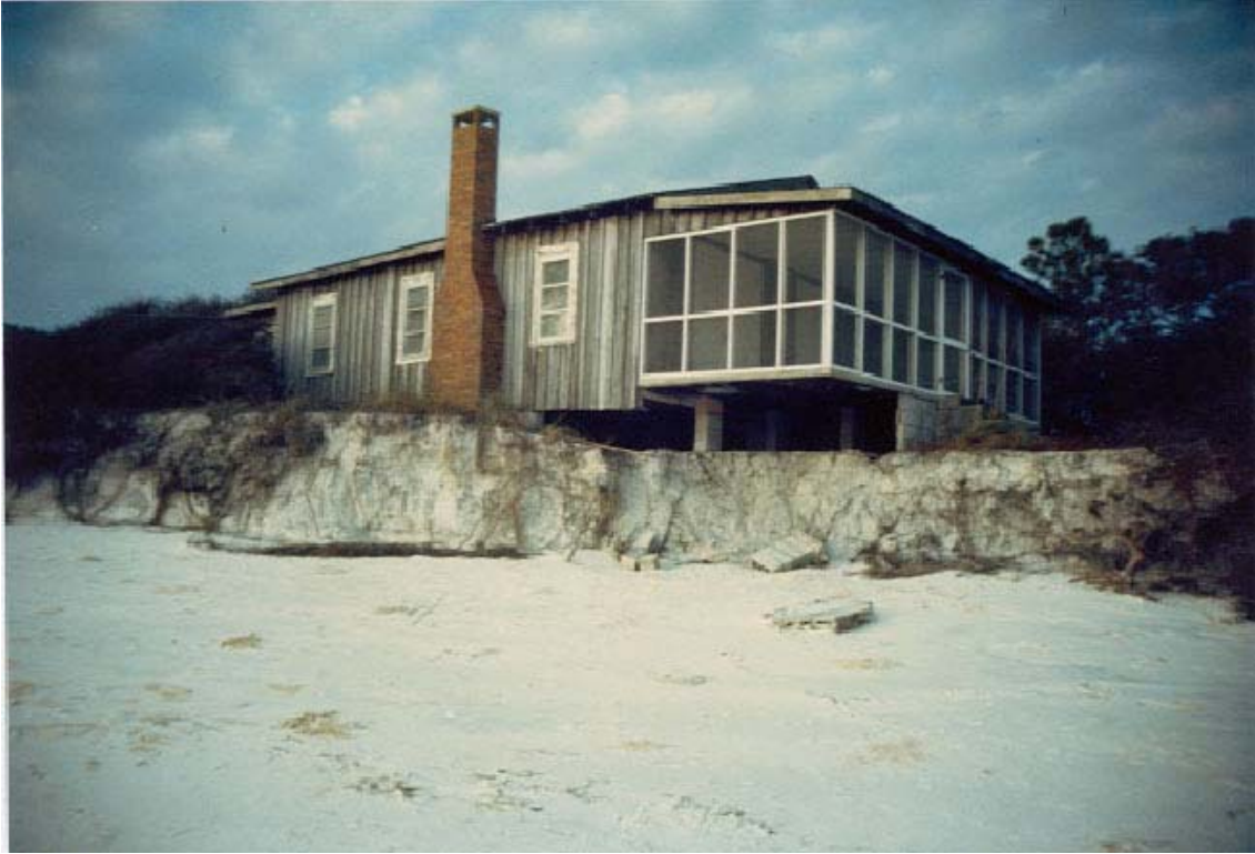
FIGURE 89. Southwest Cape dwelling partially undermined by Kate.
