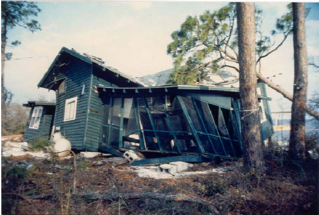
FIGURE 70. Landward side of same dwelling still supported by original grade showing the collapse in the middle.
