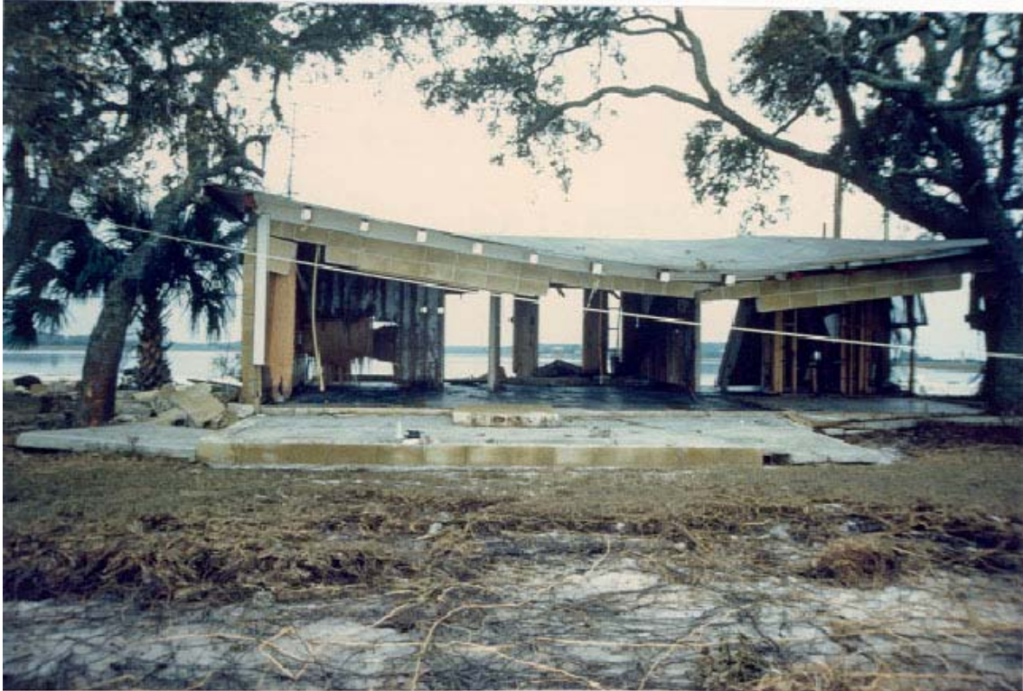
FIGURE 116. Slab-on-grade dwelling gutted by the waves and flooding.
