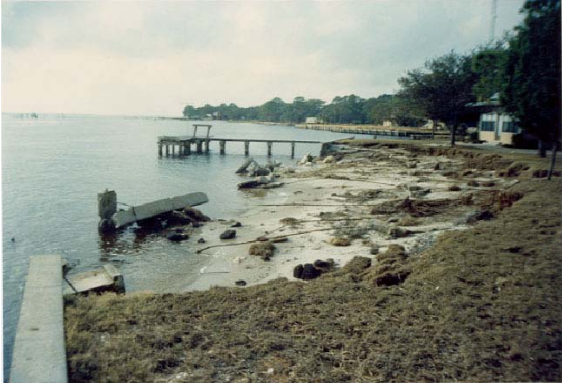
FIGURE 100. Ochlockonee Bay shoreline bulkheads destroyed at Blue Heron Way.
