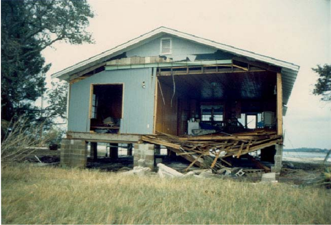
FIGURE 115. Frame dwelling on footings destroyed by wave loads.
