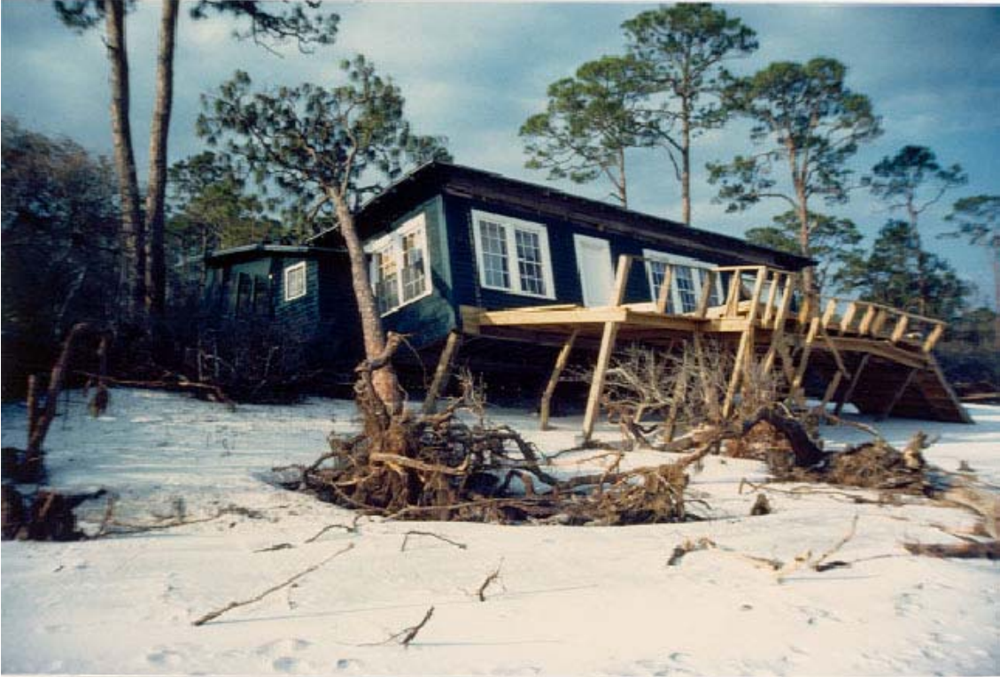
FIGURE 69. Dwelling with one front row of piles collapsed when undermined by erosion.
