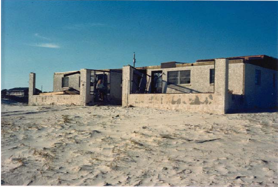
FIGURE 51. Duplex sustained major structural roof damage.
