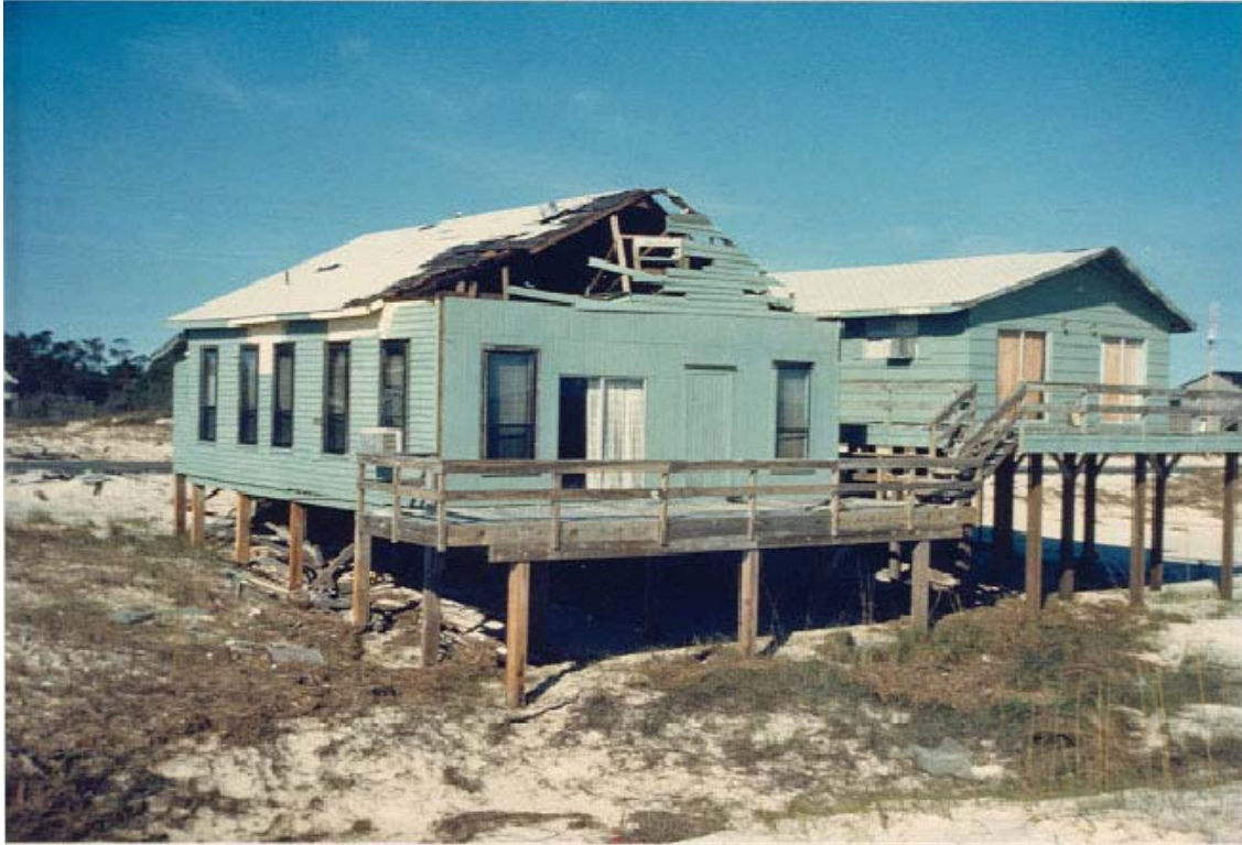
FIGURE 45. Severe Structural roof damage due to wind.
