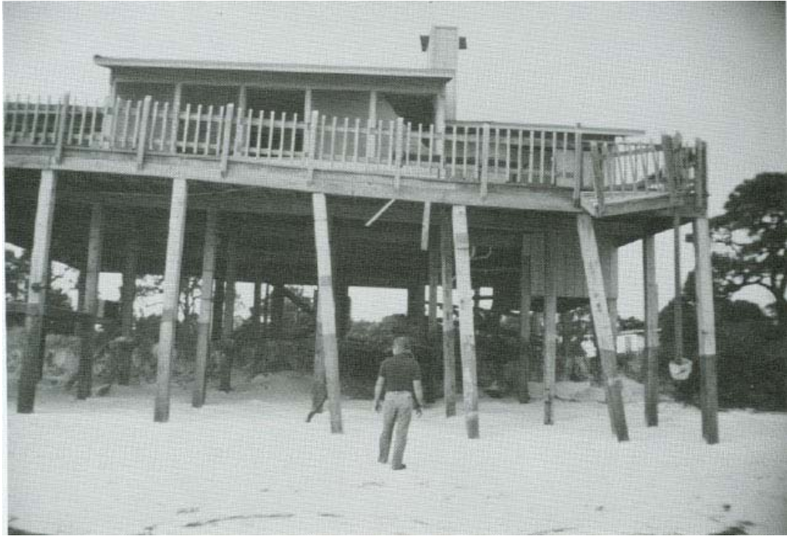
FIGURE 95. Pile-supported dwelling with insufficient pile penetration was damaged by scour.
