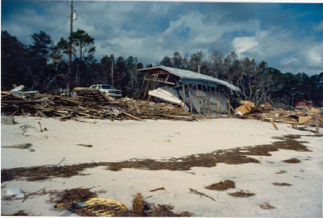
FIGURE 77. Pile-supported mobile home which survived Elena was destroyed by Kate..
