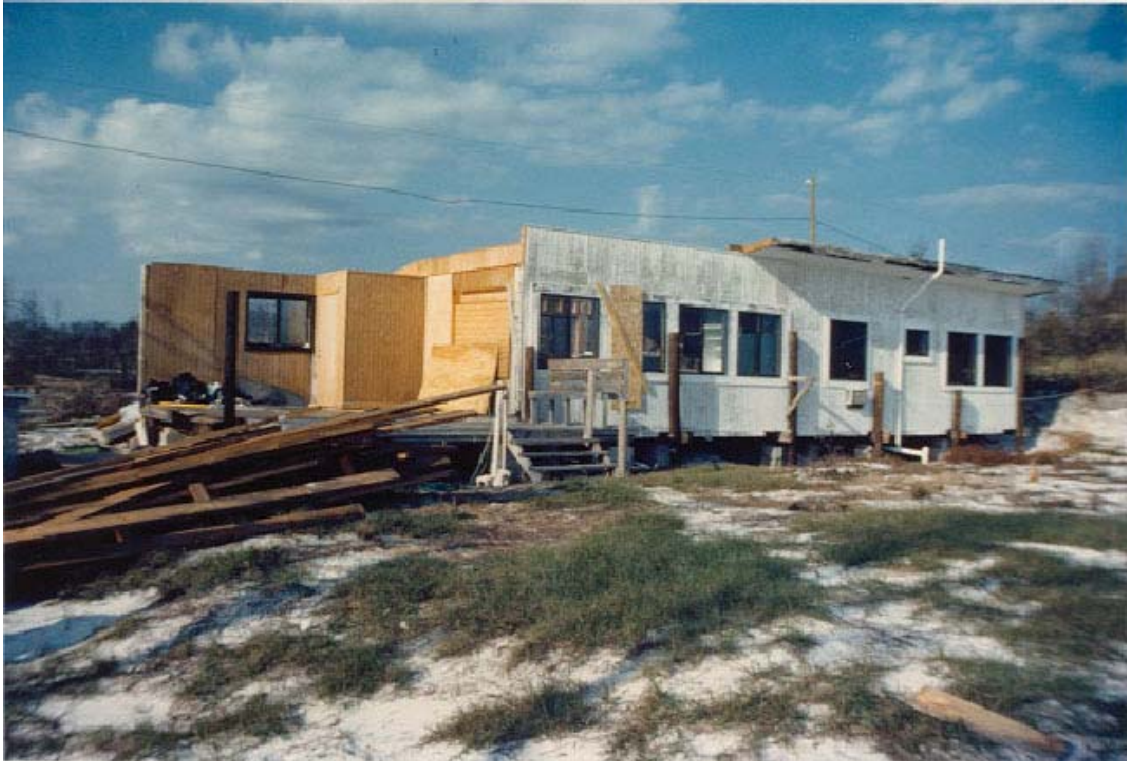
FIGURE 74. Manufactured dwelling destroyed by wind, with the roof blown across U.S. Highway 98.
