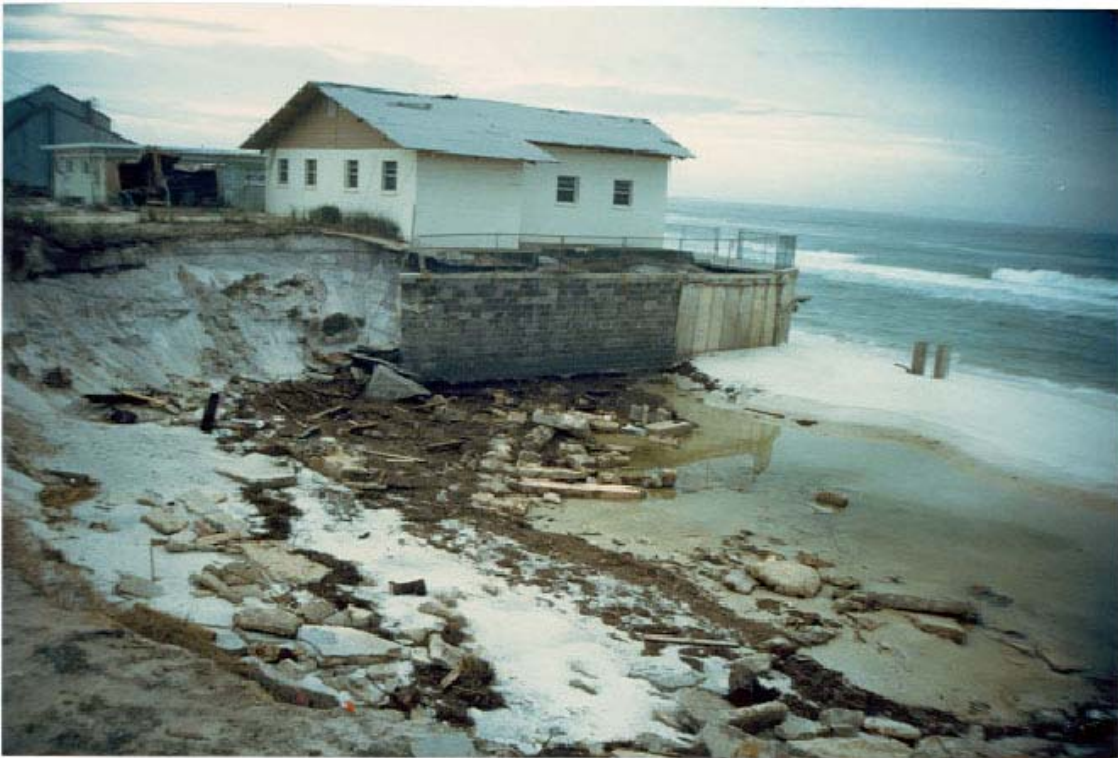
FIGURE 8. Heavy Dune Erosion adjacent Spyglass Drive has flanked a return wall and threatens a dwelling.
