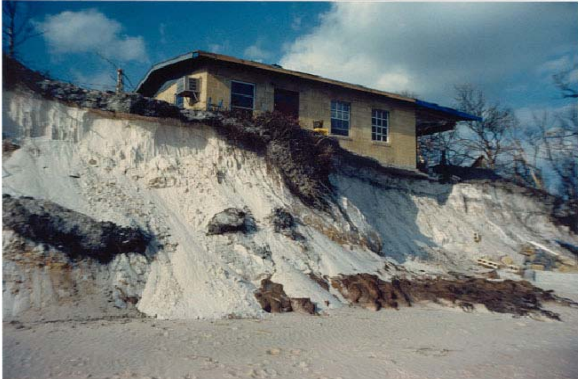
FIGURE 73. Partially undermined and damaged dwelling in imminent danger from severe dune erosion.
