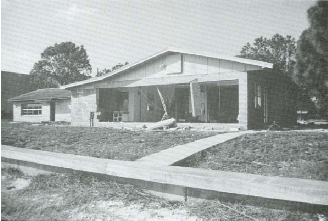
FIGURE 107. Shell Point beach dwelling damaged by waves and flooding.
