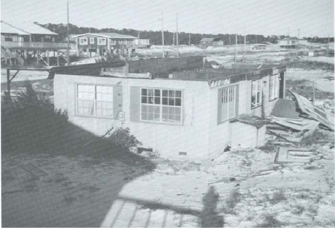
FIGURE 53. Frame dwelling damaged beyond repair by wind and wave loads.
