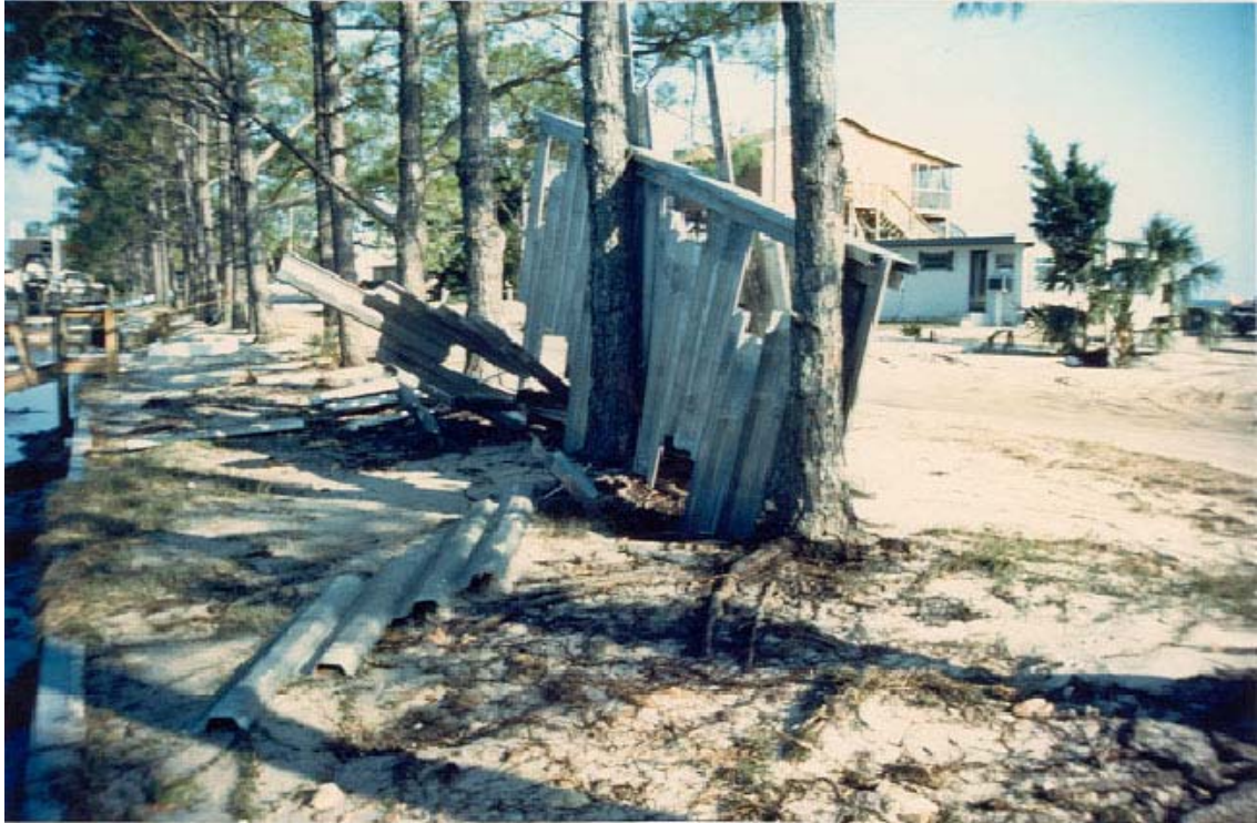
FIGURE 108. Aluminum bulkhead debris transported inland on Shell Point.
