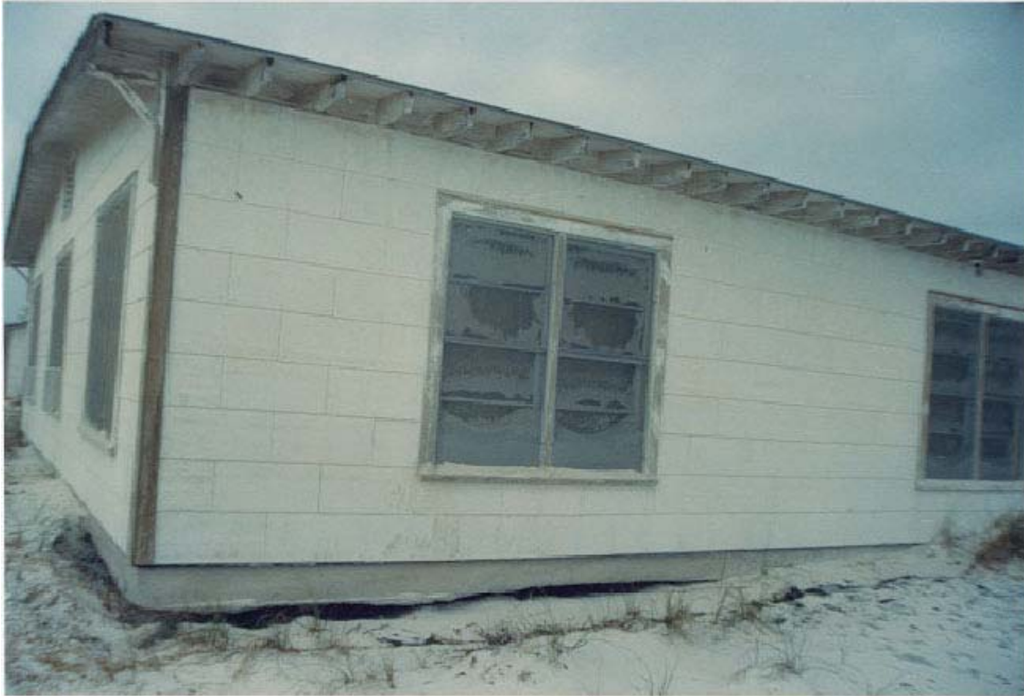
FIGURE 63. Wind undermined the slab, sandblasted the paint off the trim, and filled the screen windows with sand.
