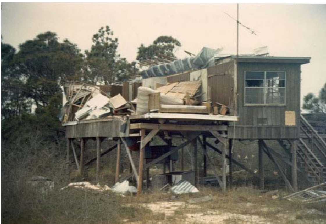
FIGURE 42. destroyed dwelling on Gulf Beach Drive.
