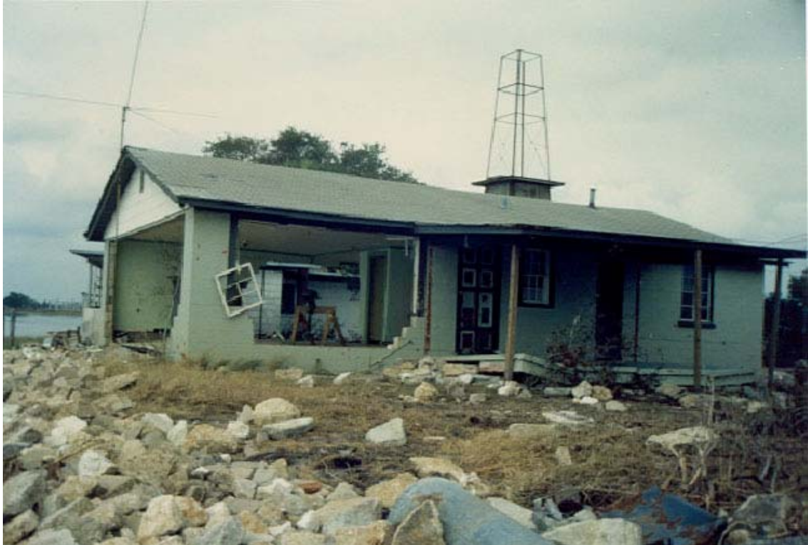
FIGURE 114. Dwelling destroyed at Walker Creek entrance.
