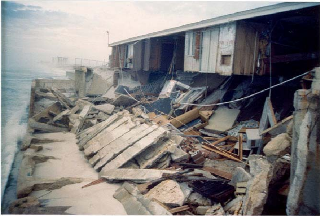
FIGURE 7. Treasure Island Motel Damage, Panama City Beach.
