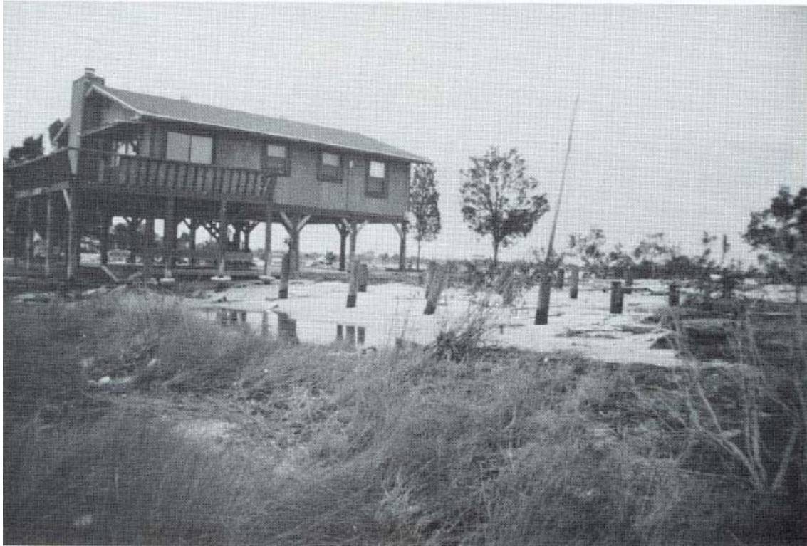
FIGURE 119. Foundation piles are sole remains of dwelling which "disappeared" during Kate.
