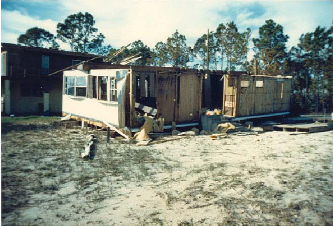
FIGURE 24. Manufactured dwelling destroyed by winds, waves, and flooding.
