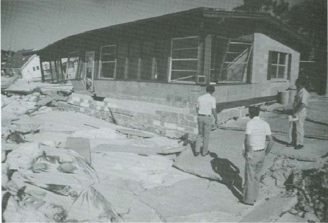
FIGURE 91. Concrete block dwelling damaged by Elena.
