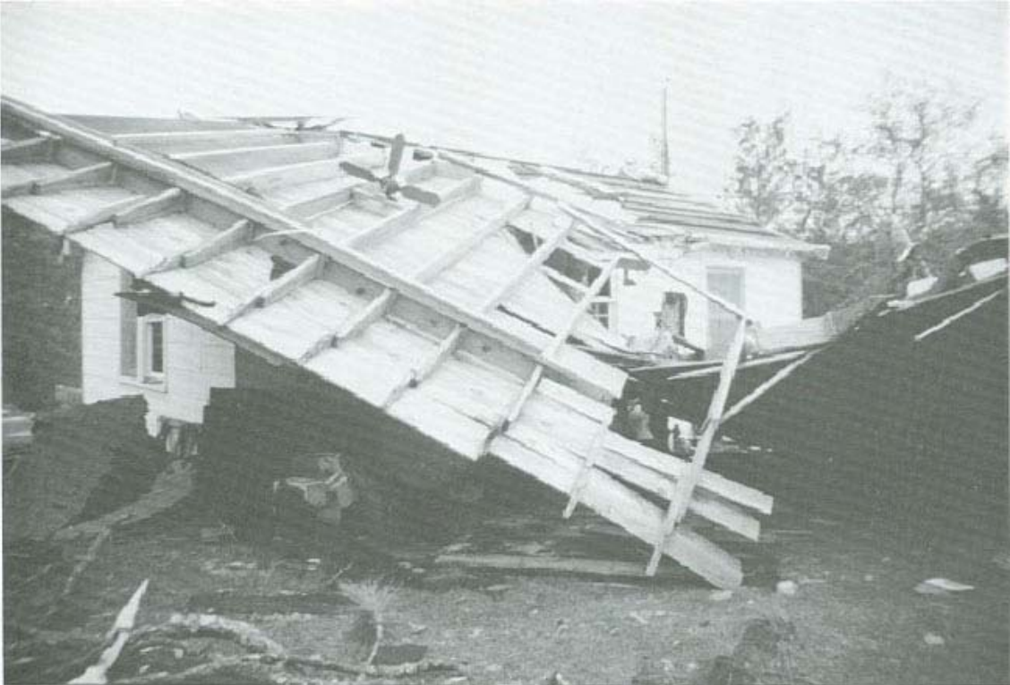
FIGURE 86. St. Teresa dwelling damaged by the impact of an airborne roof off another dwelling.
