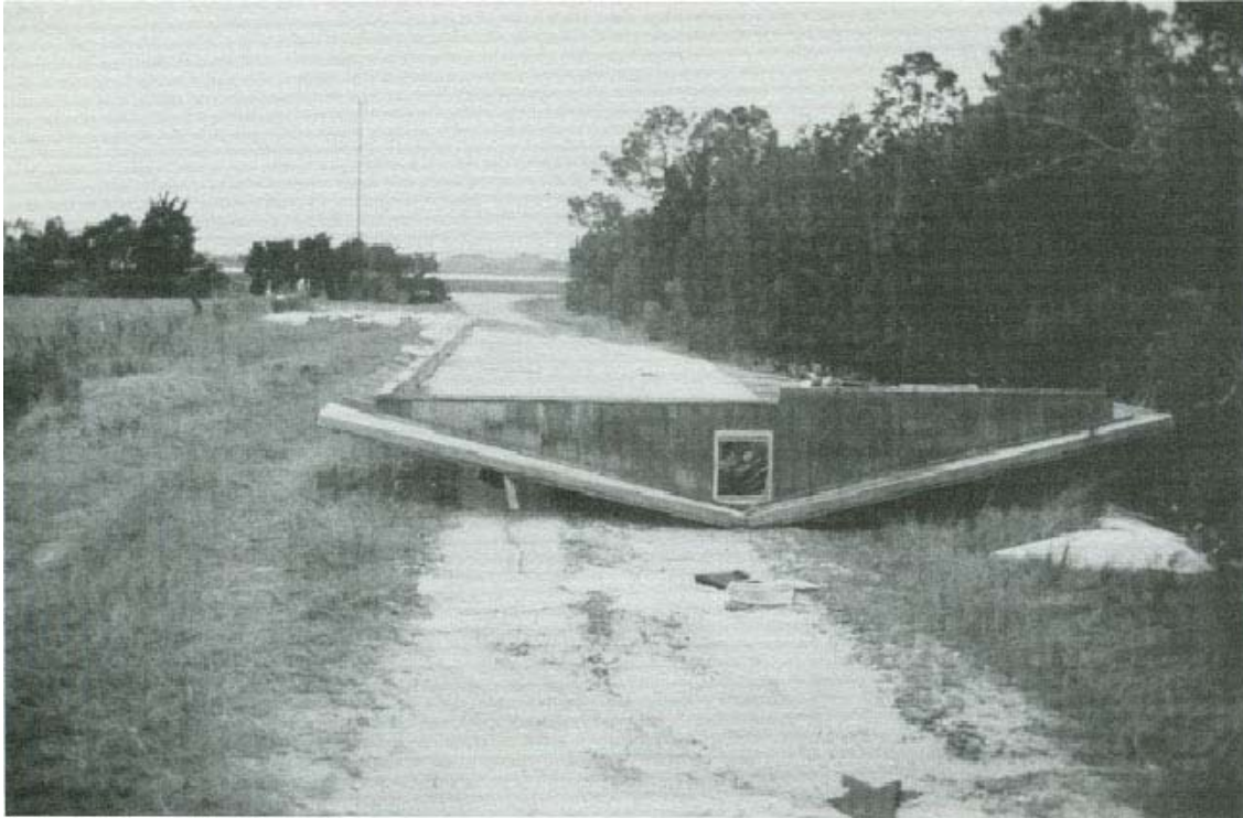
FIGURE 121. The roof was blown 1,000 feet inland and deposited in one piece on an access road.
