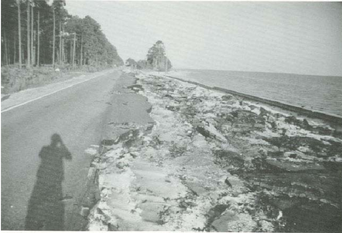
FIGURE 67. U.S. Highway 98 destroyed near Green Point.
