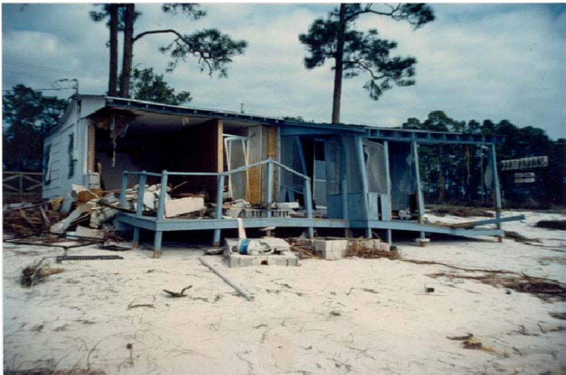
FIGURE 84. Dwelling destroyed by waves west of Martha Anns Motel.
