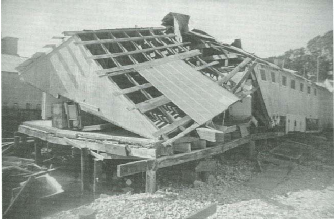
FIGURE 66. Oyster house damaged by flooding and waves, Eastpoint.
