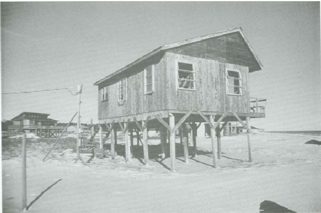
FIGURE 50. Pile-supported dwelling with inadequate pile to beam connections and insufficient pile penetration leans following wind loads and scour.
