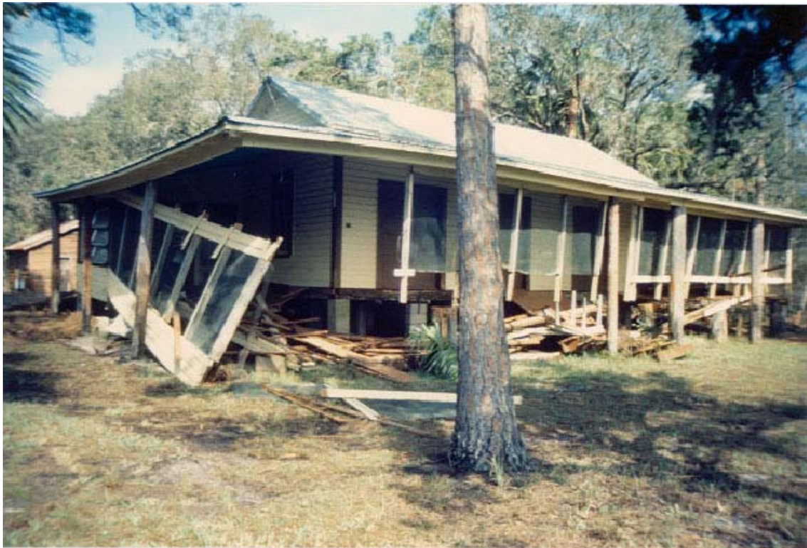
FIGURE 109. Beach dwelling damaged by waves and flooding.
