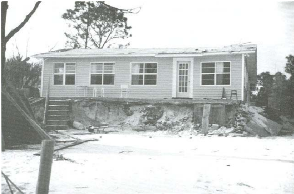
FIGURE 71. Dwelling threatened by erosion, St. George Sound shoreline.
