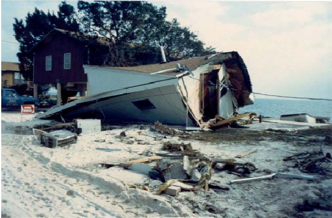
FIGURE 117. Grade level frame dwelling destroyed by waves.
