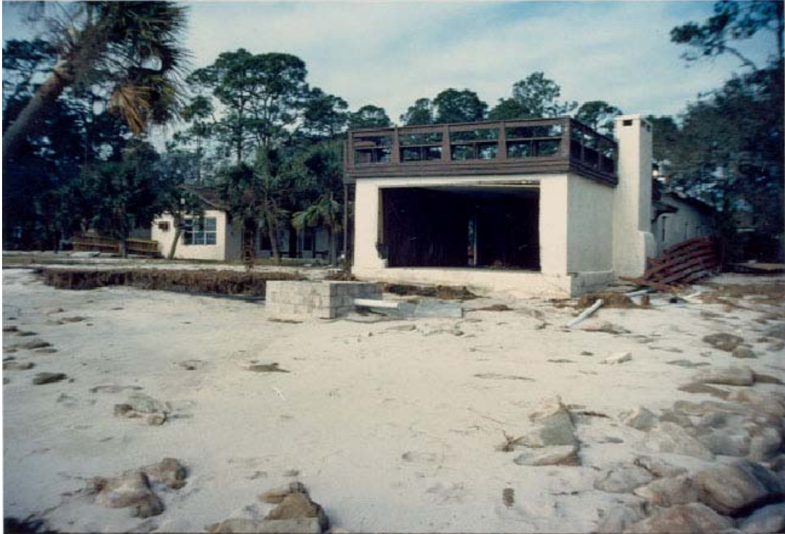
FIGURE 83. Wave loads damaged seaward unit of motel St. James.
