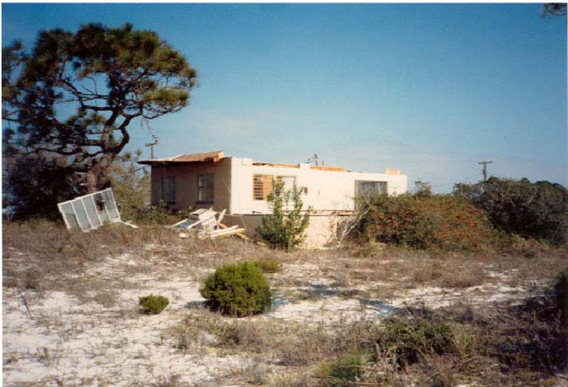
FIGURE 88. Flat roof blown off Alligator Point dwelling.
