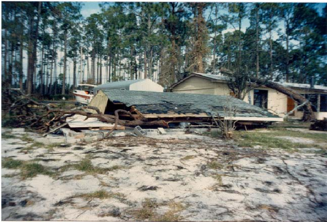
FIGURE 82. Wind and wave loads destroyed a St. James structure.
