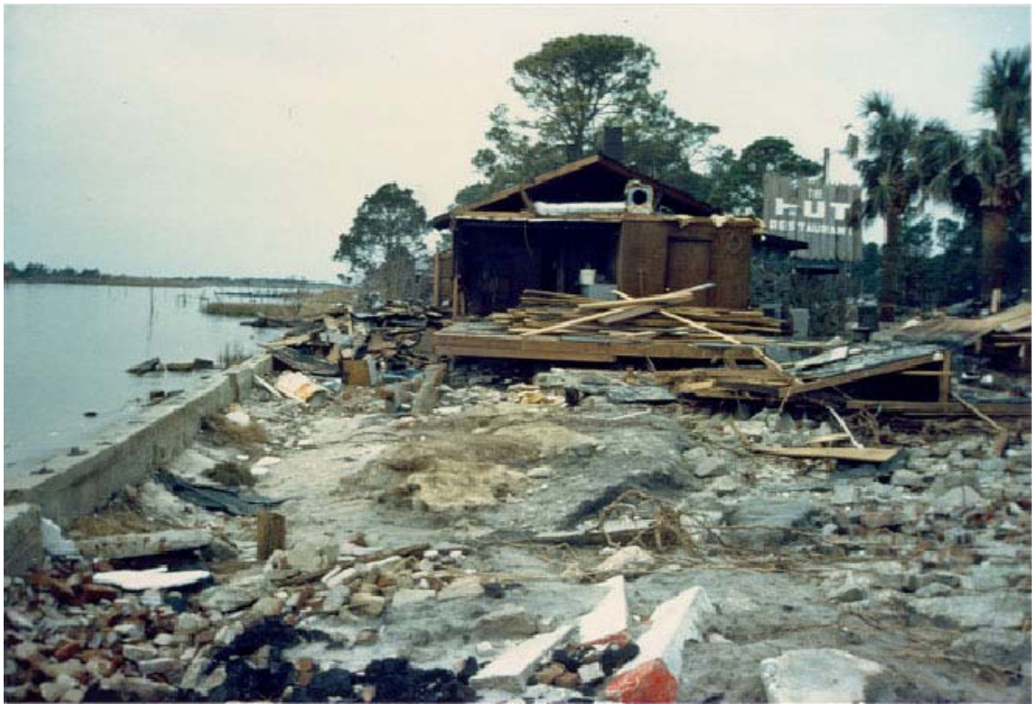
FIGURE 33. Wave damage to the Hut Restaurant on Apalachicola Bay shoreline.
