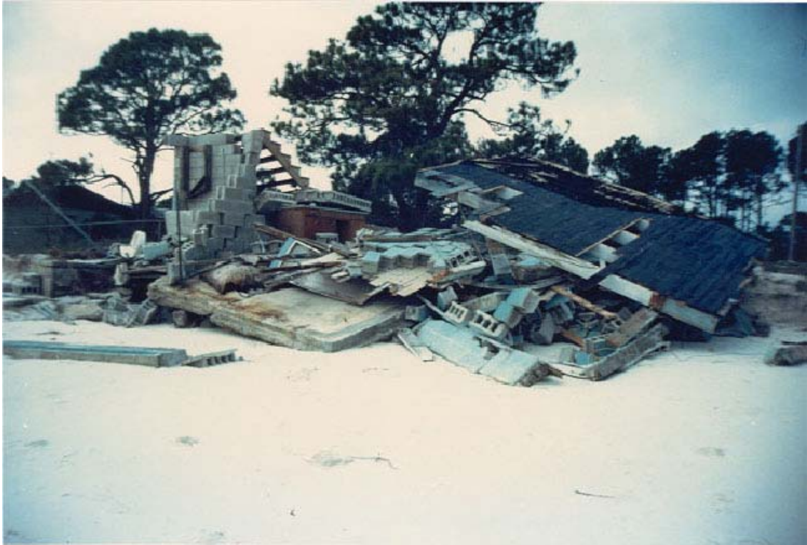
FIGURE 94. Concrete block dwelling destroyed by wave loads.
