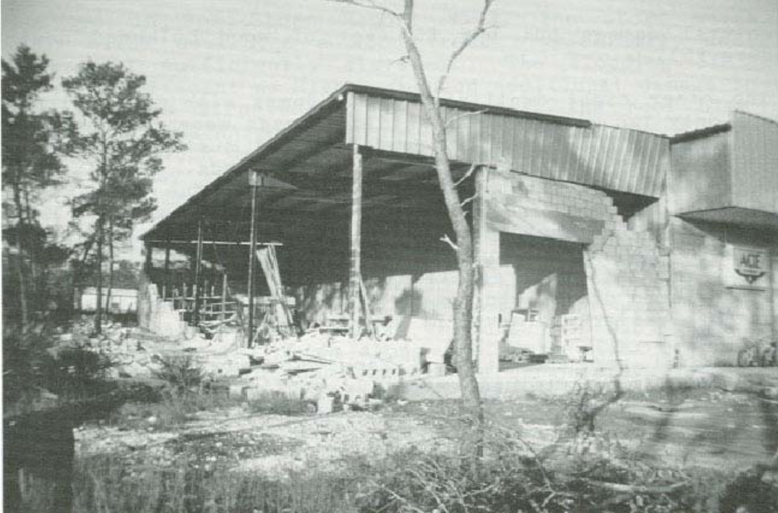
FIGURE 65. Ace Hardware store damage by wind, Eastpoint.
