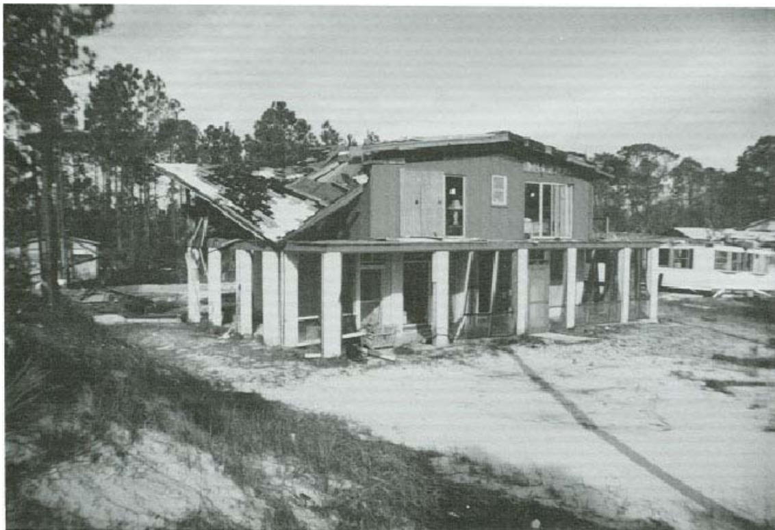
FIGURE 23. Dwelling damaged by wind and flooding.
