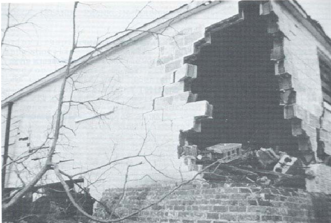
FIGURE 36. Building damaged by waves at the mouth of the Apalachicola River.
