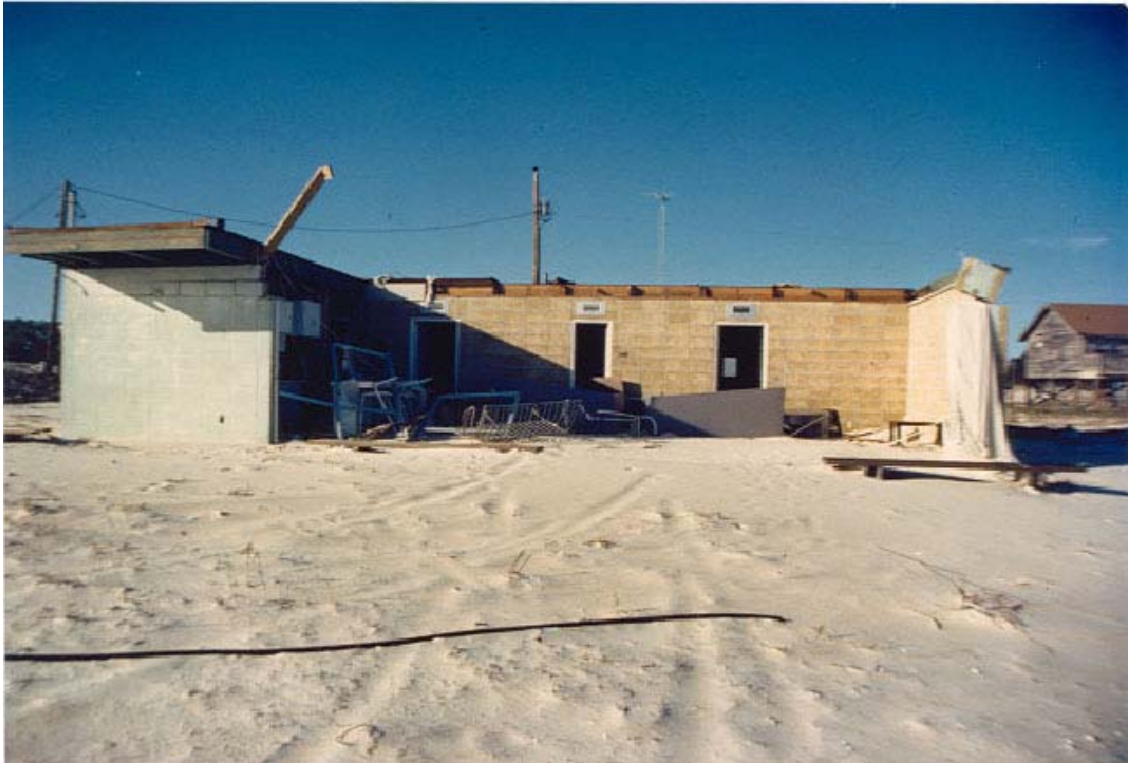
FIGURE 52. Dwelling with roof blown off and seaward wall destroyed by waves.
