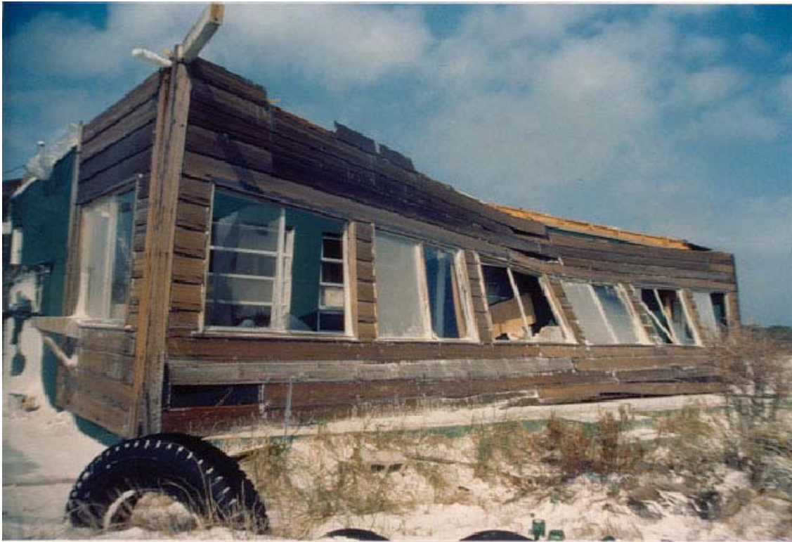
FIGURE 64. Island dwelling with heavy wind damage.
