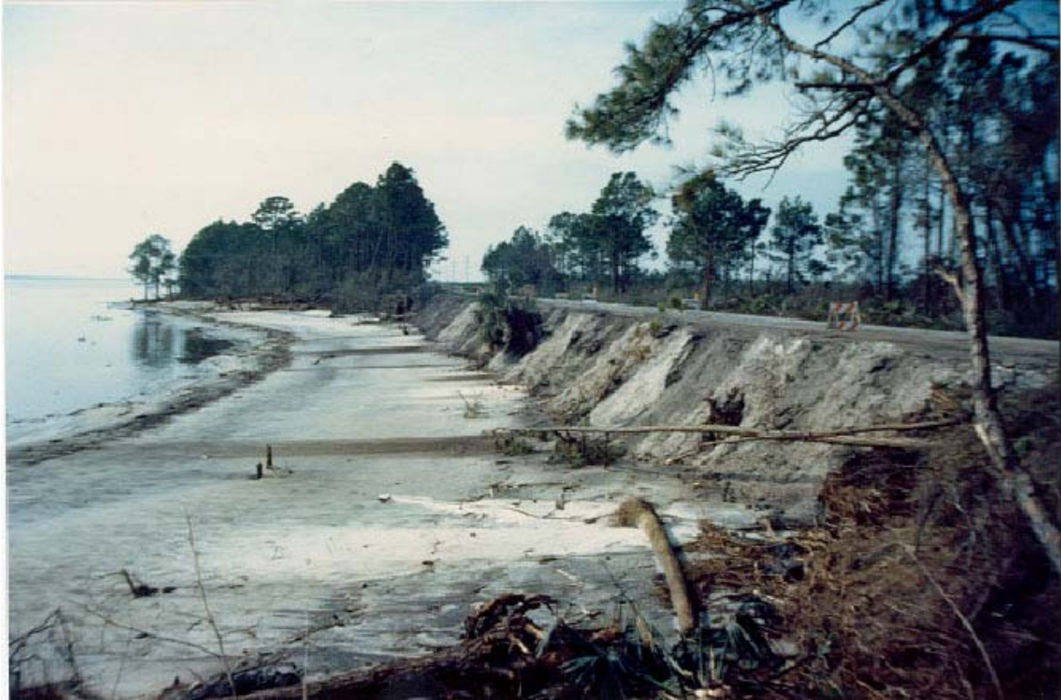
FIGURE 28. Franklin County Road 3022 damage from St. Vincent Sound shoreline erosion.
