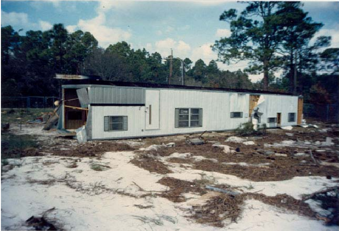
FIGURE 75. Mobile home rolled over by the wind and flooded.
