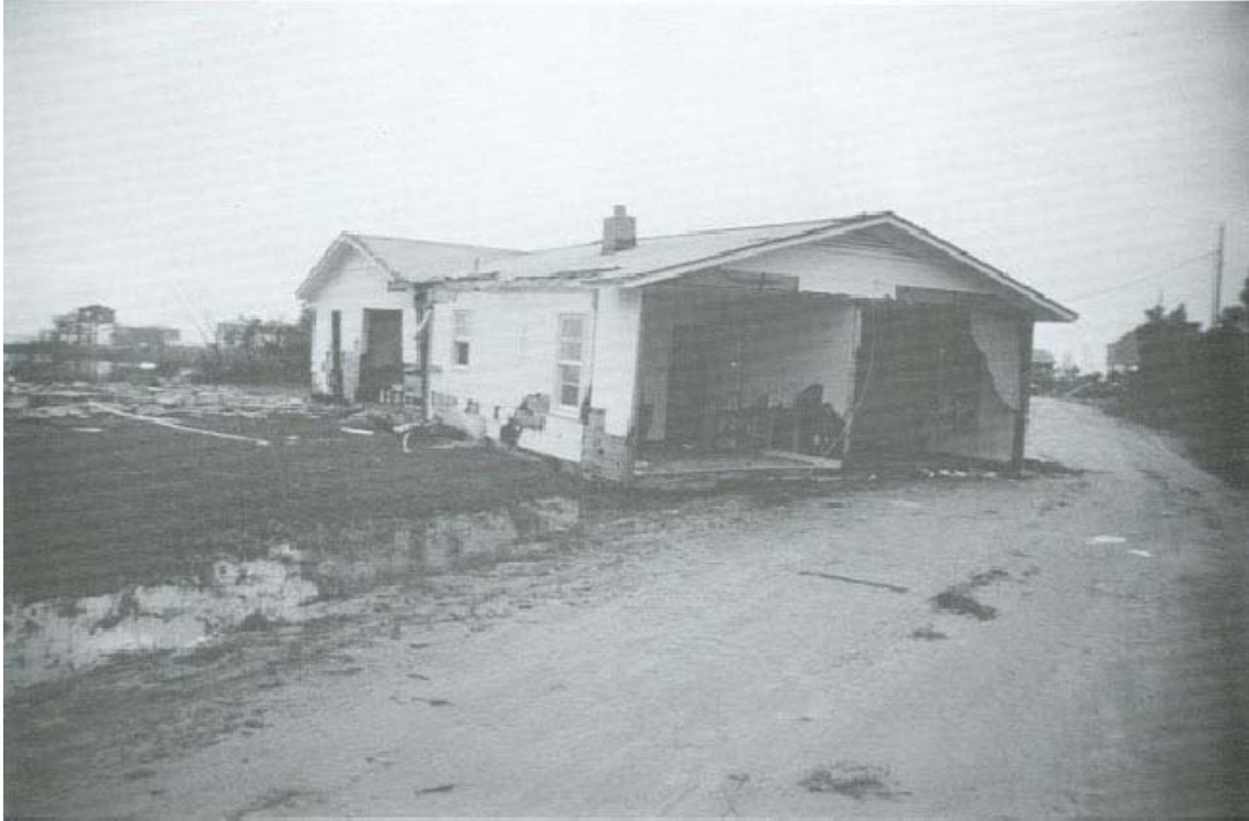
FIGURE 104. Oyster Bay dwelling damaged by waves, floated inland by flood waters, and deposited on road.
