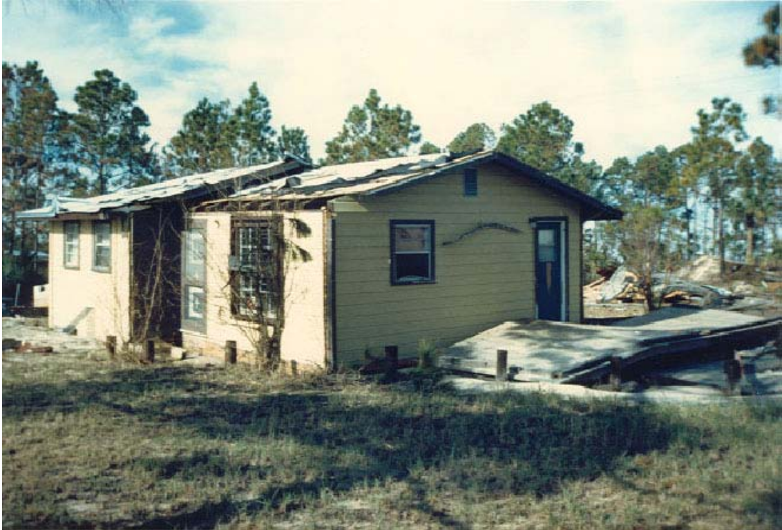
FIGURE 25. Damaged dwelling floated off its short pile foundation.
