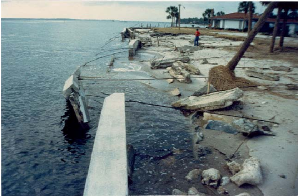
FIGURE 101. Bulkheads destroyed at Sunrise Lane on Ochlockonee Bay.
